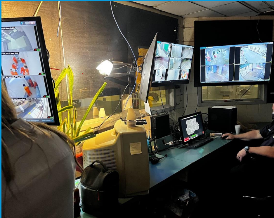
Main Control Room
